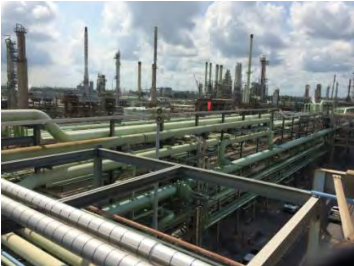
Fig. 2. Photograph Showing a Portion of Existing Exaggerated 3-Story Tall Pipe Racks Subject to Expansion (Courtesy of Fluor Corporation)
